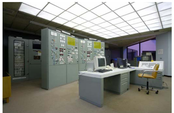
The control room at Wivenhoe Power Station
